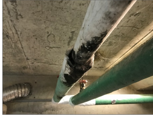
Photo 8 - Mouldy/stained pipe insulation in Beaver/Otter Pump Room
