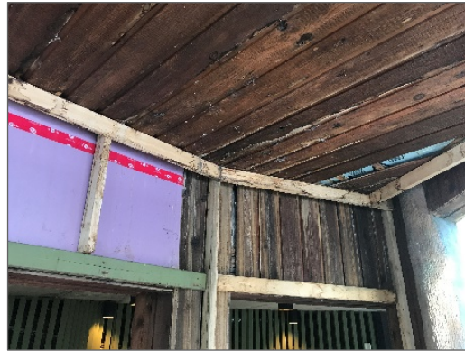
Photo 6 - Mouldy/water damaged wood ceiling and bulkhead wall in Otter Viewing area
