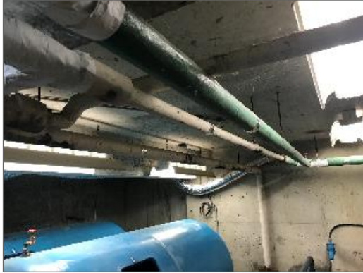
Photo 7 - Mouldy/stained pipe insulation in Beaver/Otter Pump Room
