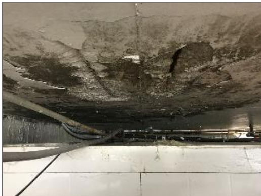
Photo 1 - Mould growth and eroded concrete ceiling above Walk-in Cooler in the Basement
