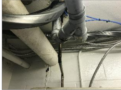
Photo 4 - Mouldy/water damaged pipe Insulation in Fountain Drink area
