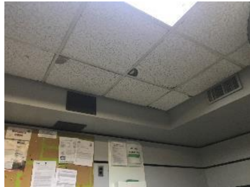
Photo 2 - Water damaged/mouldy ceiling tiles in the Staff Room
