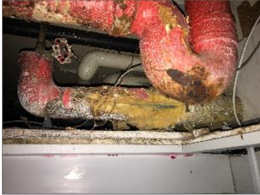
Photo 3 - Mouldy pipe insulation in ceiling space in the Staff Room
